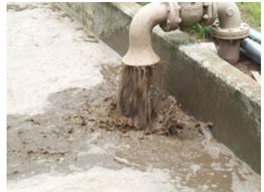
Wasting at an Activated Sludge Facility
